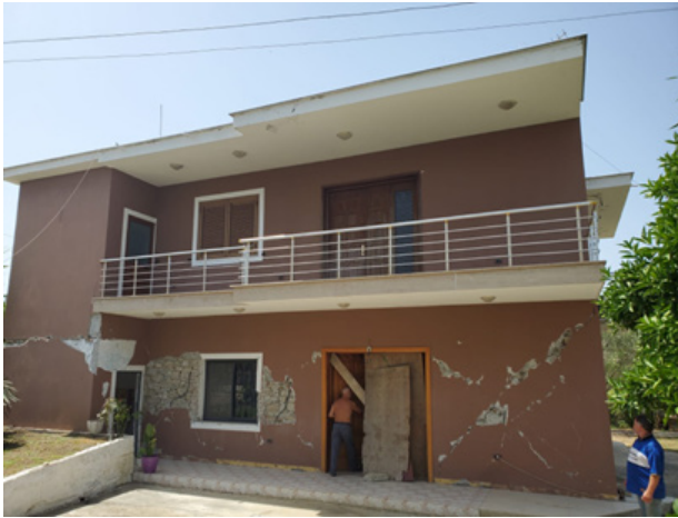
Figure 2. Building A diagonal shear cracks on perimeter wall
