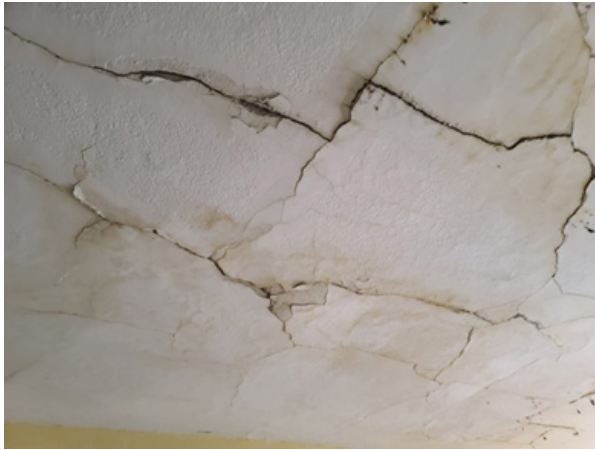
Figure 3. Building B slab degradation and separation from walls
